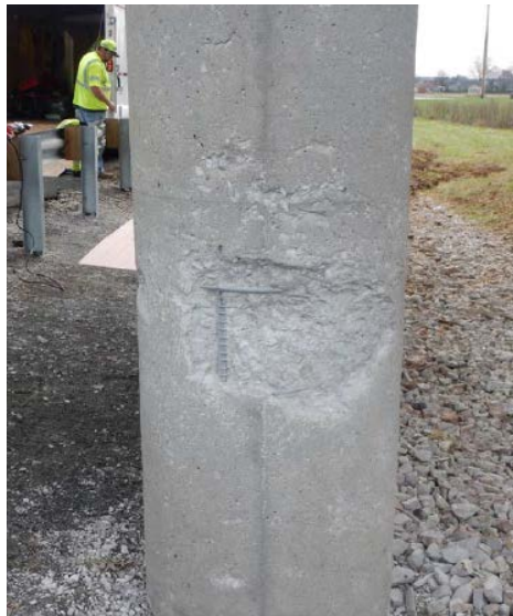
(a) Impacted area of column
